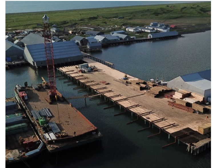
Peter Pan's Port Moller plant was damaged by a 2017 fire and rebuilt in 2018. Reconstruction and upgrades of the plant are examples of processors' investment in Alaska.
